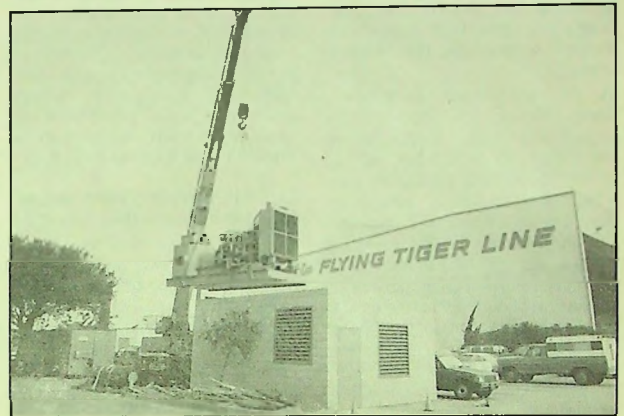
A Caterpillar 800 kilowatt diesel generator was installed at Flying Tigers headquarters recently to provide a back-up source of power in the event of a commercial power outage. The standby generator, shown above as it is lifted by a 40-ton hydraulic crane into the blockhouse where it will be stationed, will provide back-up power to all computer and communications equipment in the Information Systems Computer Center and the Operations Control Center.
